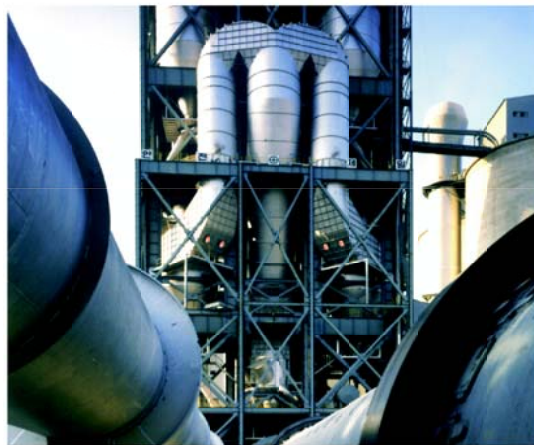
VSR BLASTER® air cannons in a cement plant (Foto: Krupp Polysius)
